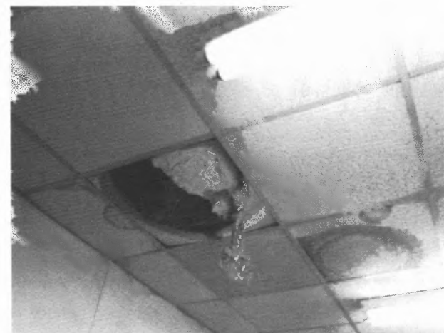
Unrepaired roof. "The roof has been a problem for a long time. There is water dripping through the roof. This has been mended numerous times, but not well enough, and the problems returned."
